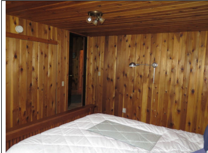
ABOVE: Another view of the bedroom but looking toward the living room area. (1151)
